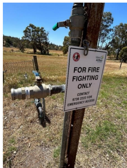
Quindanning standpipe couplings
