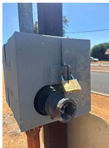
Lock to access standpipe
