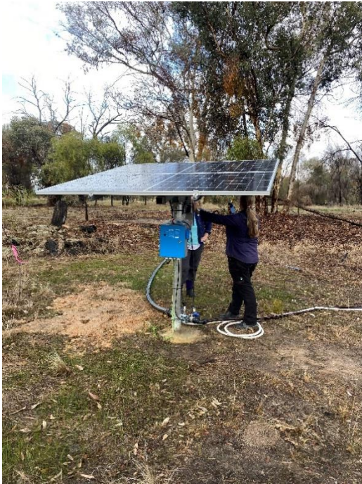
Solar panel and pump
