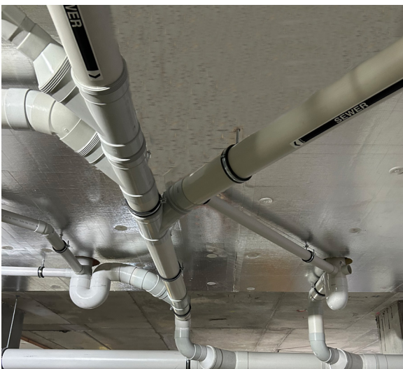
Photo 1: Typical EDP pipework
