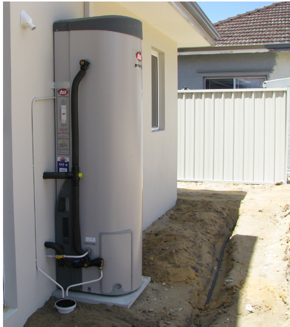
Photo 2: Typical insulation requirements on a storage water heater
