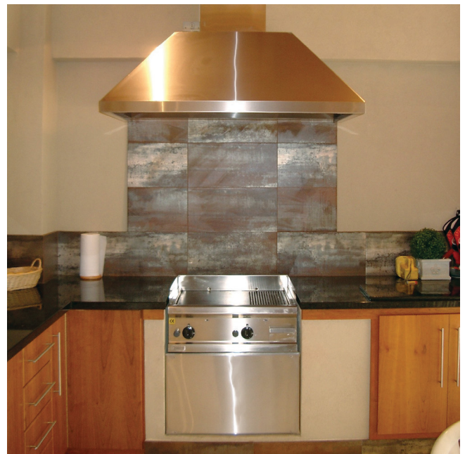
A commercial gas barbecue with mechanical ventilation.
