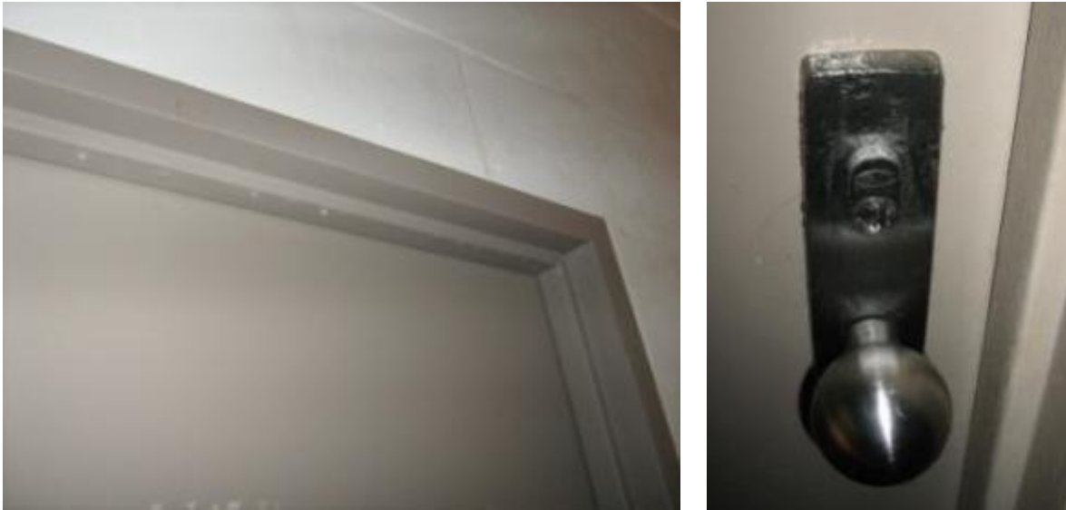
Figure 8 Condensation on outside face of door, frame and hardware due to cold tracking from cooled space
