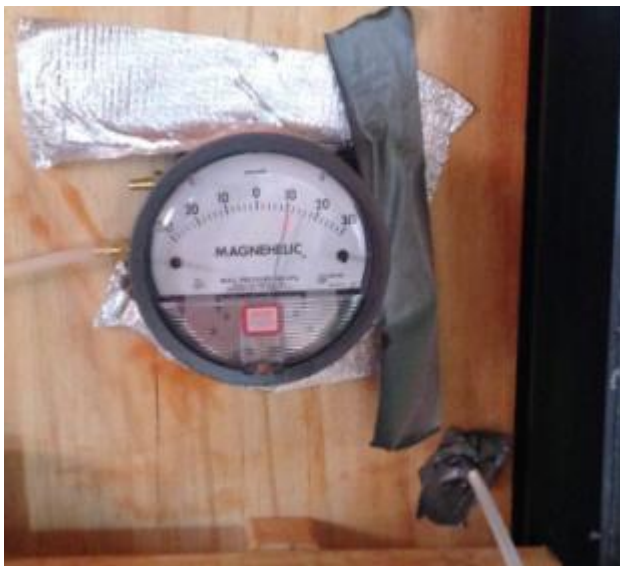
Figure 33 Fit pressurisation fan into a doorway and install pressure-sensing meter to read inside and outside air pressures.
