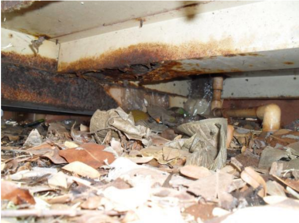
Figure 4 Vegetation and wind-blown debris accumulate easily under and around external mechanical equipment
