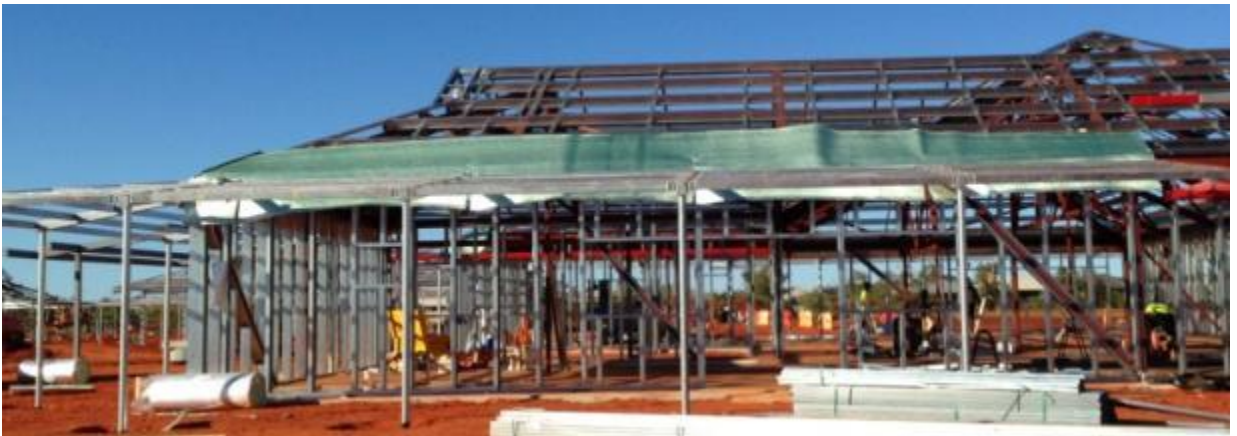
Figure 21 The continuity of the vapour barrier between the wall and the roof must be maintained
