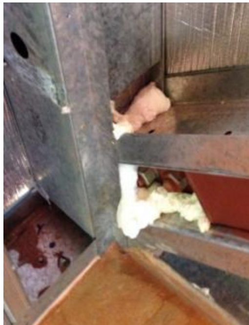
Figure 28 Seal hard-to-reach gaps in the barrier with expanding foam filler e.g. at corners where multiple frame members limit access. Gaps in the barrier can be identified by daylight leaking through, and reflecting on the barrier material.
