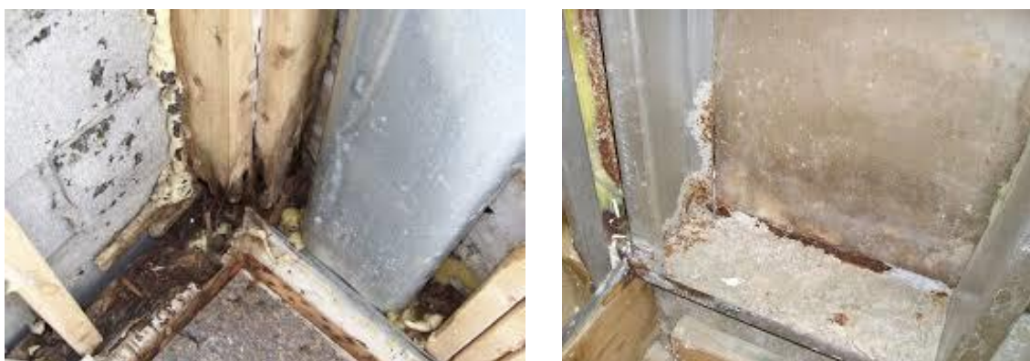
Figure 11 Corrosion in framing due to moisture retention in wall panel
