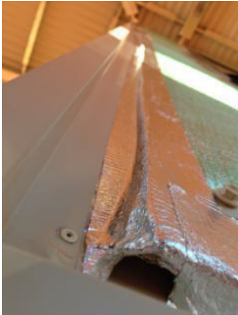
Figure 31 Carefully inspect the barrier to find points of weakness such as ends of flashings where the continuity of the seal is broken. Seal any breaks found, where possible, with adhesive tape or expanding foam as appropriate.
