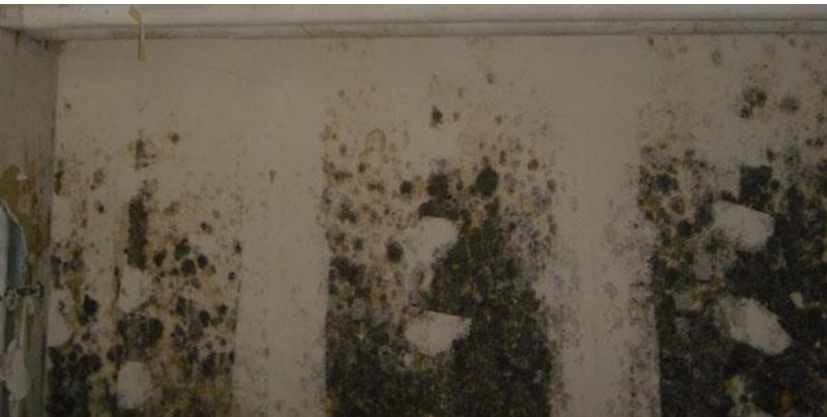
Figure 7 Mould formed in wall sheeting saturated by condensation
