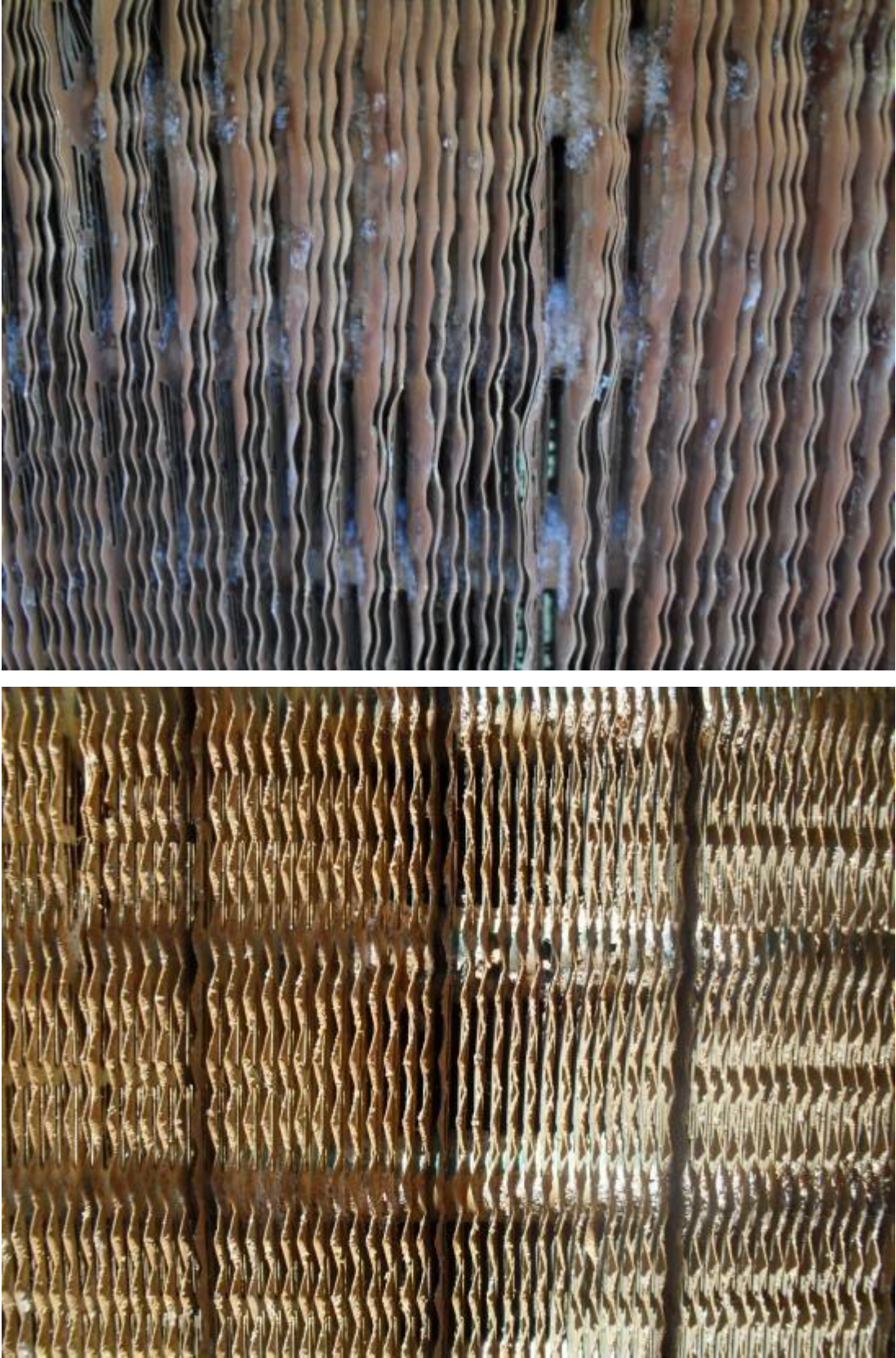
Figure 17: Example of fins with salt deposits on tubes and fins.
