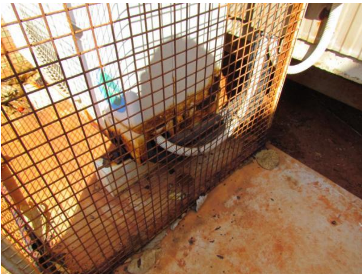
Figure 3 Example of corrosion frequently found in external units
