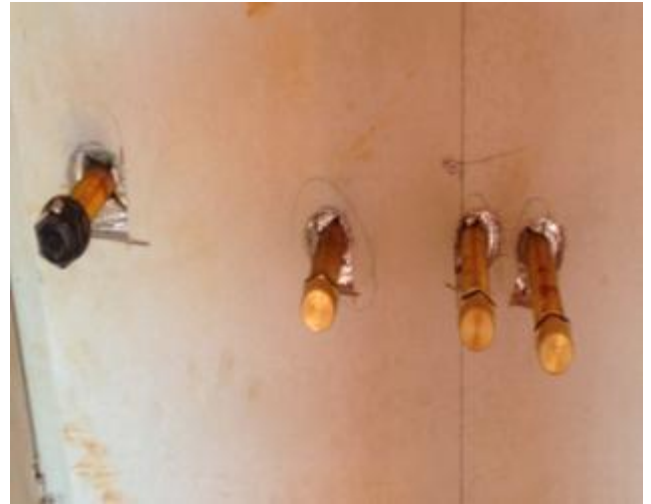
Figure 30 ABOVE AND LEFT: Seal individual service penetrations to both the inside and outside of the vapour barrier using adhesive tape
