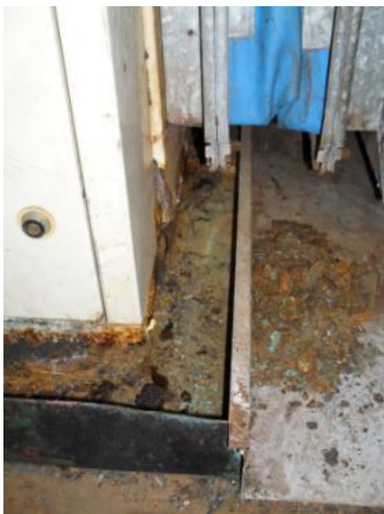
Figure 16 Corrosion caused by condensation. Insufficient insulation on equipment mounted in a ceiling resulting in condensation and corrosion. This is prevented by adding more insulation to the outside of the cabinet.
