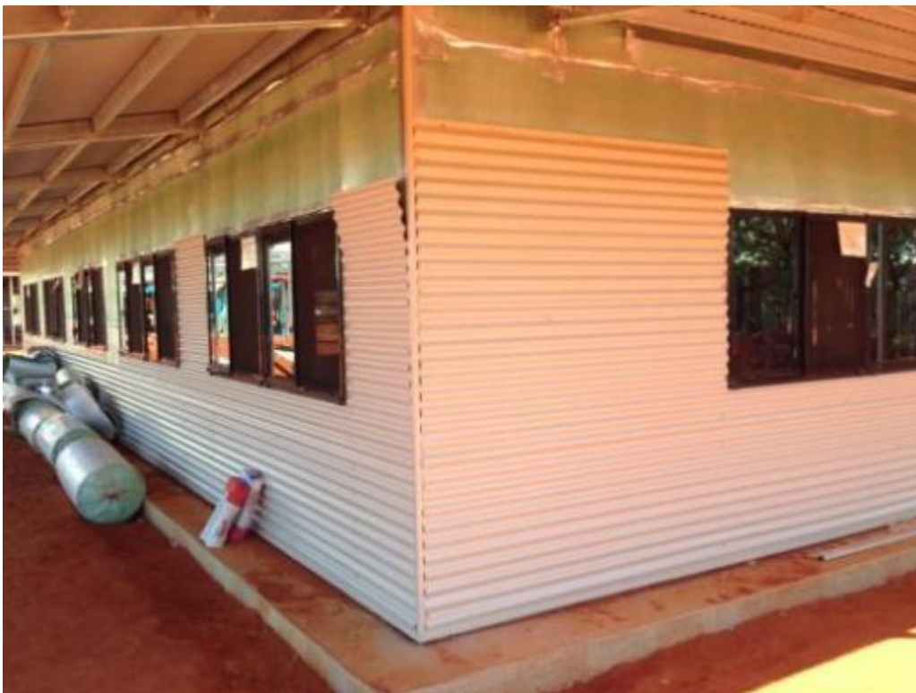
Figure 24 Wall vapour barrier should extend from bottom plate to join with the roof vapour barrier to provide a continuous seal
