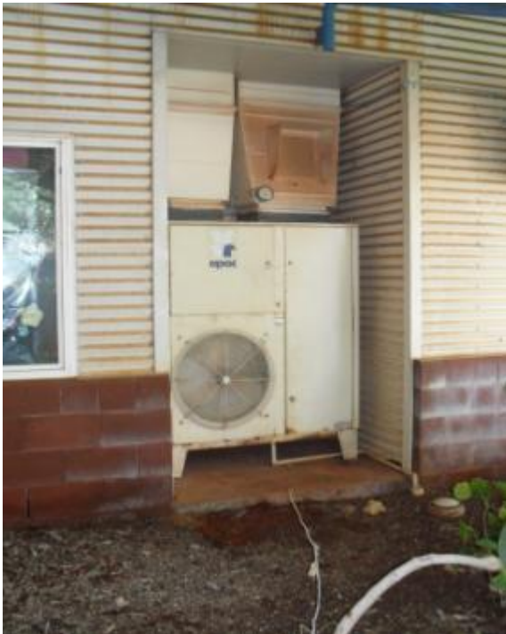
Figure 18 Cramped position of equipment limits air flow and impedes access for service
