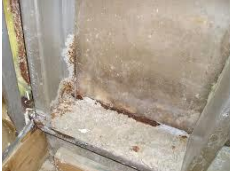
Figure 9 Evidence of interstitial condensation in wall
