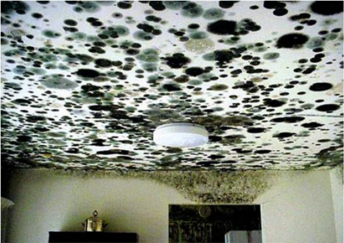
Figure 6 Mould on ceiling formed from condensation dripping from un-sarked roof above
