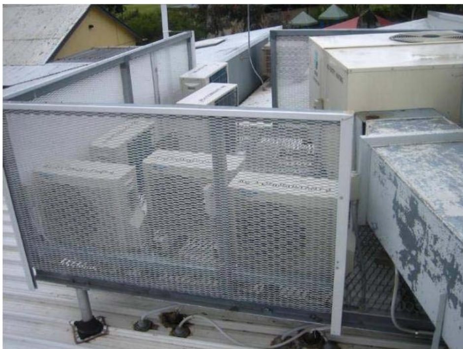
Figure 8: Example of poorly accessible mechanical equipment
