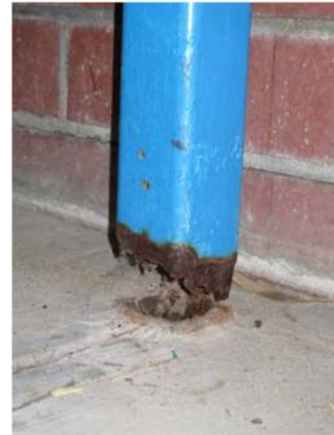
Figure 7: Potential effects of poor corrosion protection.
