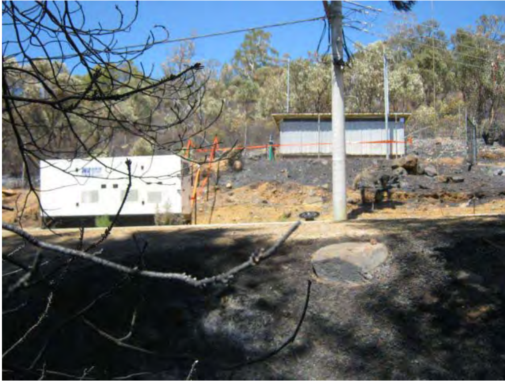
Photo 4 - Scott Road Pump Station post-fire (note supplementary generator front left)
