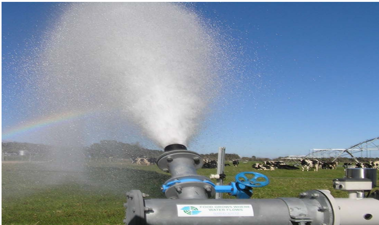
Photo 1: Water under gravity pressure in the WHID Pipe System
