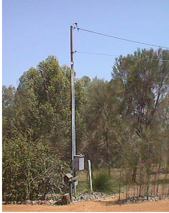
Aerial cable - rural setting
