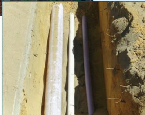
The use of a purple-pipe system to supply an alternative fit-for-purpose water source for irrigation (courtesy of the Satterley Property Group)
