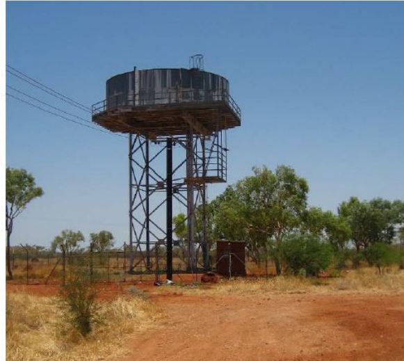
Figure 2 – Elevated water tank on SL-lot 54
