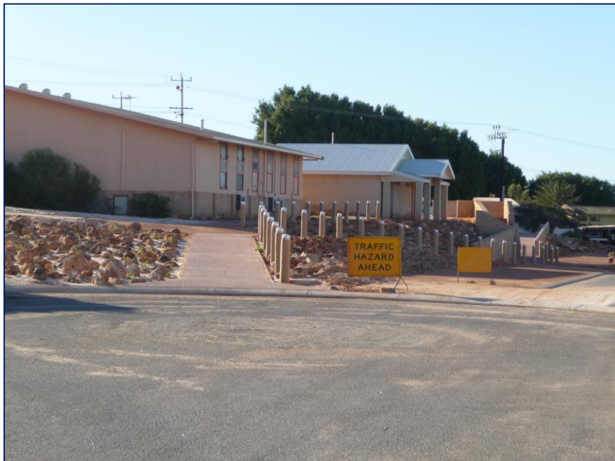
New ramped pathway and retaining walls recently constructed to link Barnard Street and Hughes Street. Landscaping has been planted and ropes along the bollards will be installed signage in Knight Terrace (July 2010)
