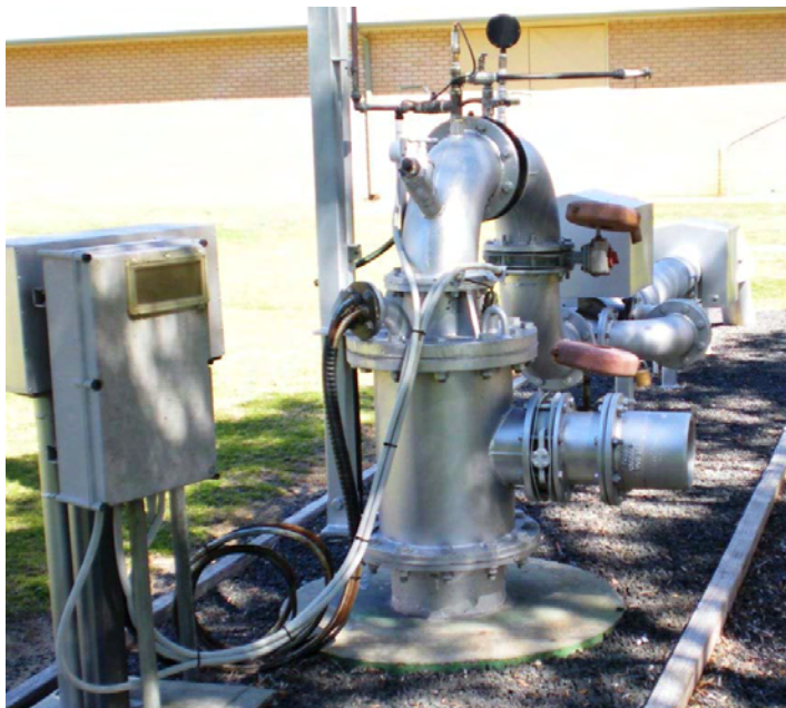
Figure B2 Bore BWB 14 at treatment plant 2 (photo: Busselton Water)
