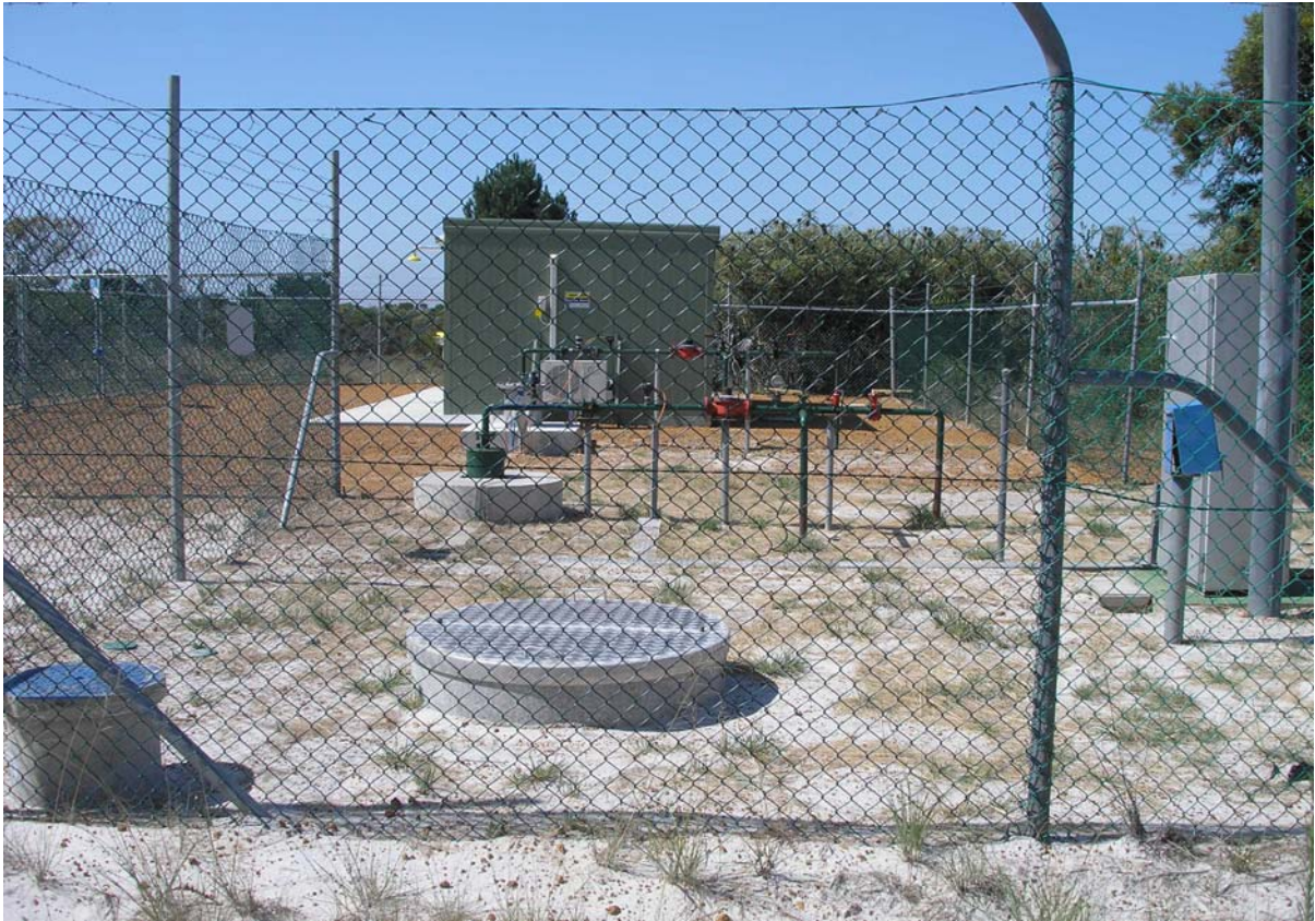
Photo 1 Compound for the Gibson drinking water supply wellfield
