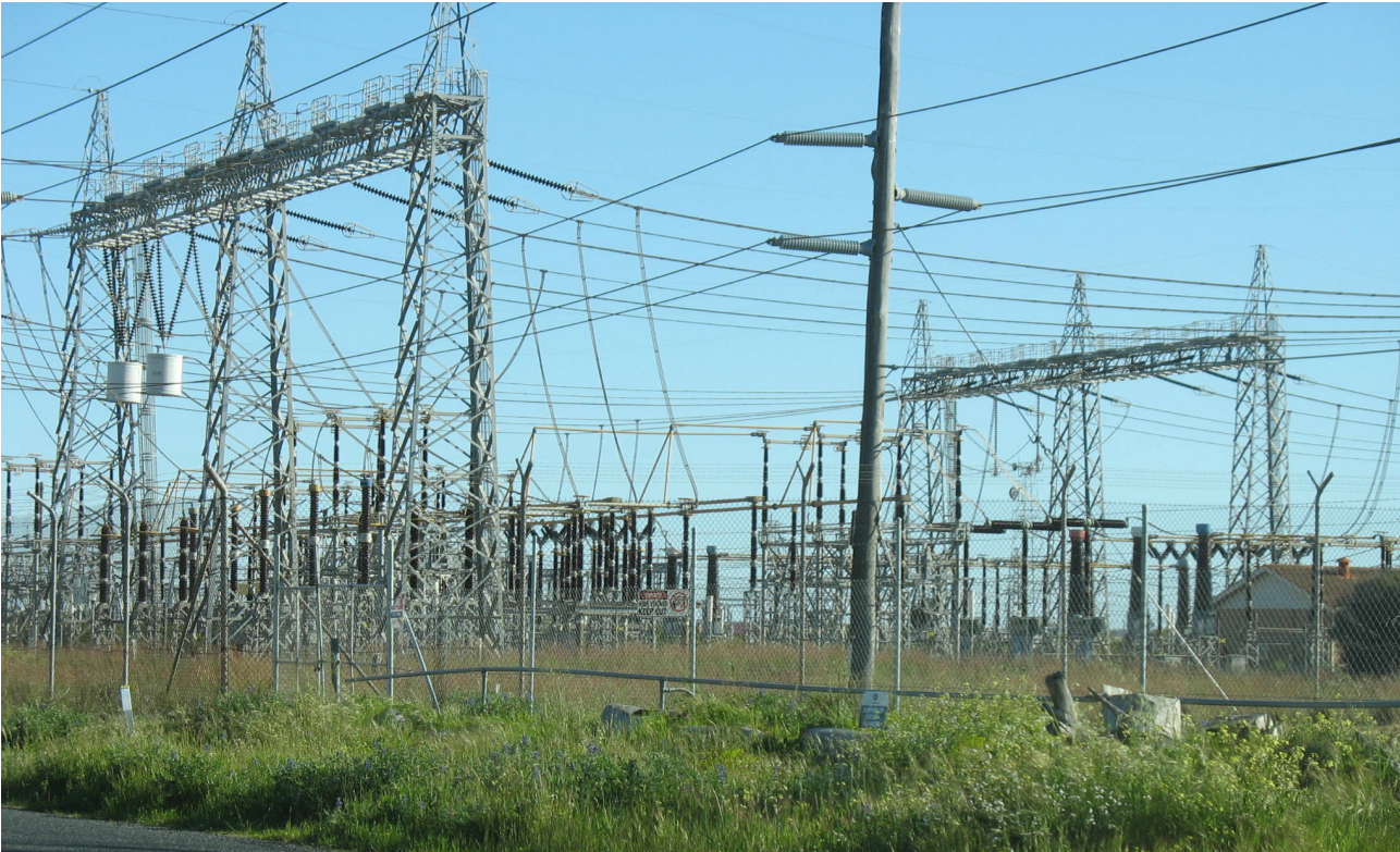
Photo. 23 Western Power substation - Malaga Public Purpose Reservation Precinct 69
