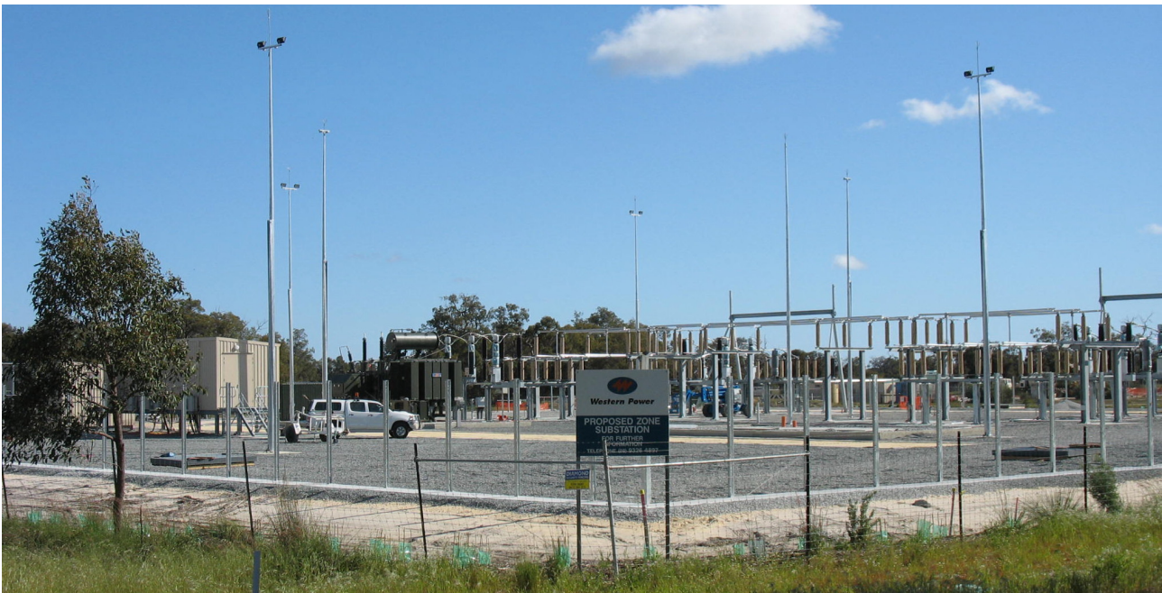
Photo. 15 Western Power Ellenbrook substation – Whiteman - proposed Public Purpose Reservation Rural Zone Precinct 74
