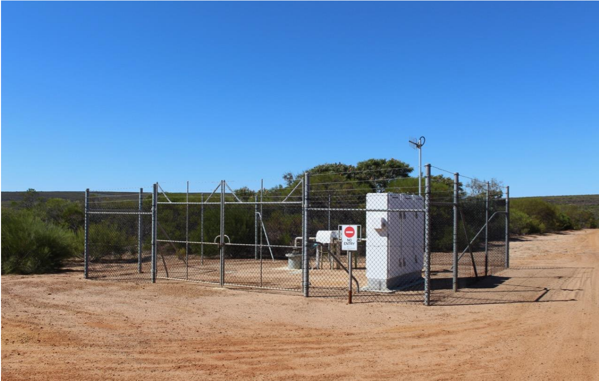
Figure C2 Fenced and locked bore compound at Port Kalbarri, photograph by J. King, DWER
