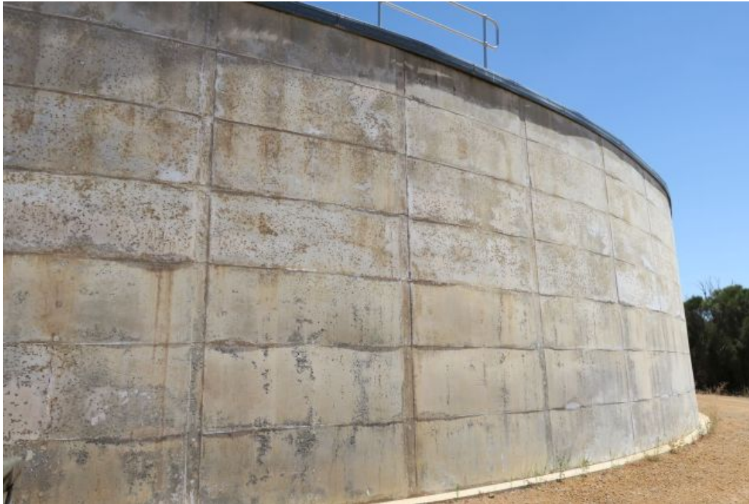
Figure C3 Water storage tank within the Katanning Catchment Area
