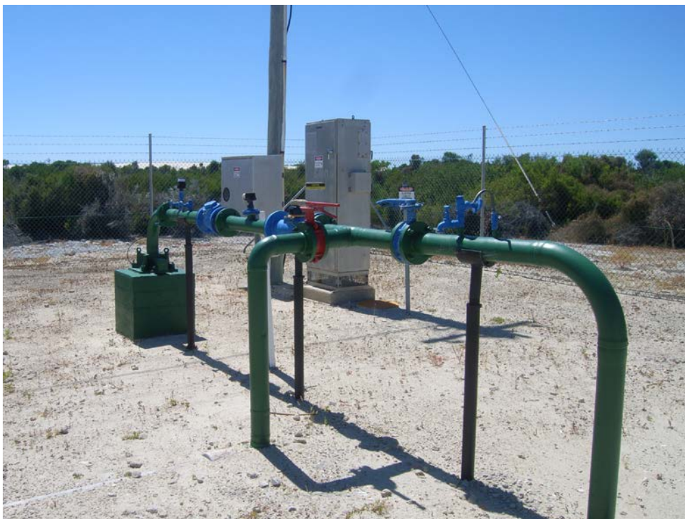
Figure C4 Production bore 3/81, photograph by J. King, Department of Water
