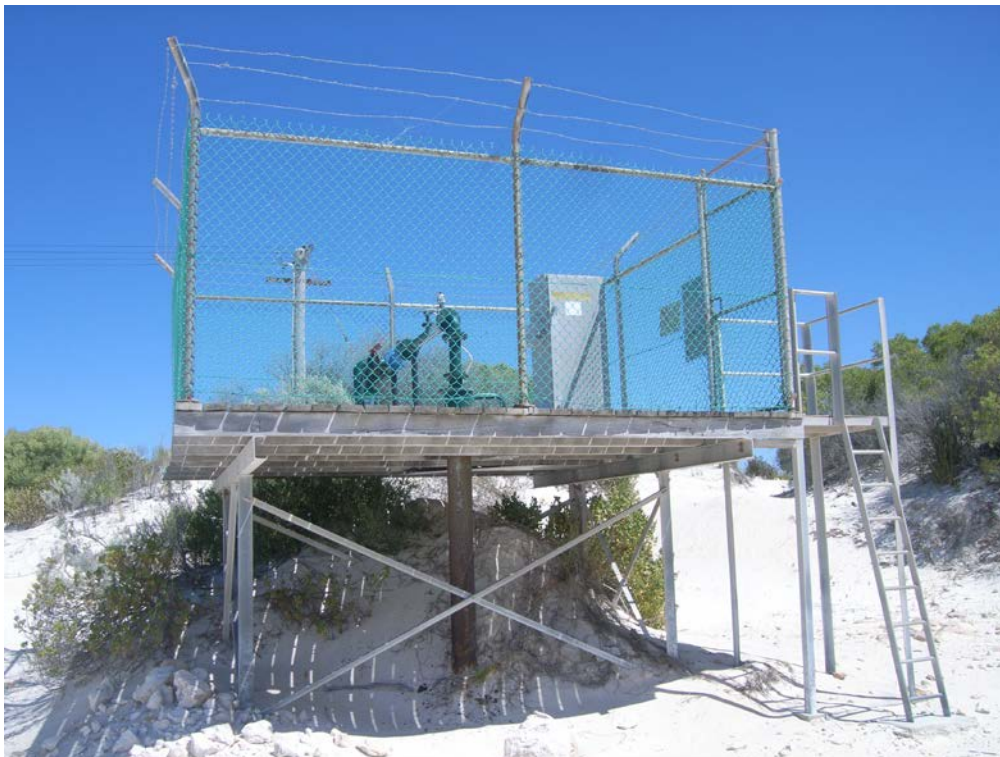
Figure C2 Production bore 2/74, photograph by J. King, Department of Water
