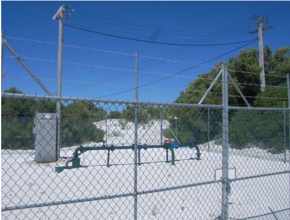
Figure C1 Production bore 2/65, photograph by J. King, Department of Water
