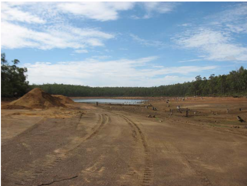
Figure B2 Mungalup Dam showing low water levels due to dam construction. Note evidence of four-wheel driving on banks (photograph taken by Kellie Clark)
