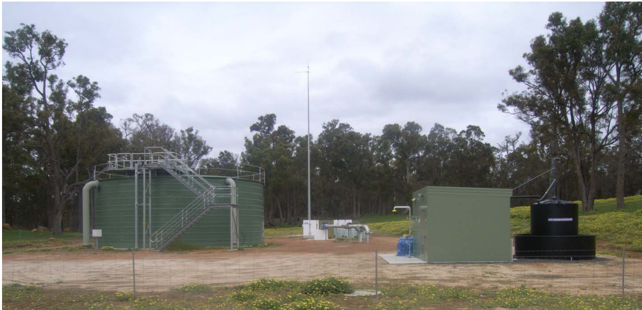
Figure C2 Nannup production bore 1/07 compound viewed from the eastern side
