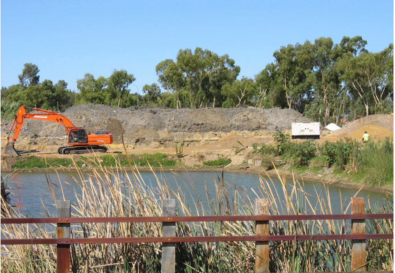
Photo. 15 Ex stables and market garden being prepared for urbanisation - Gwelup Urban Zone Precinct No 92
