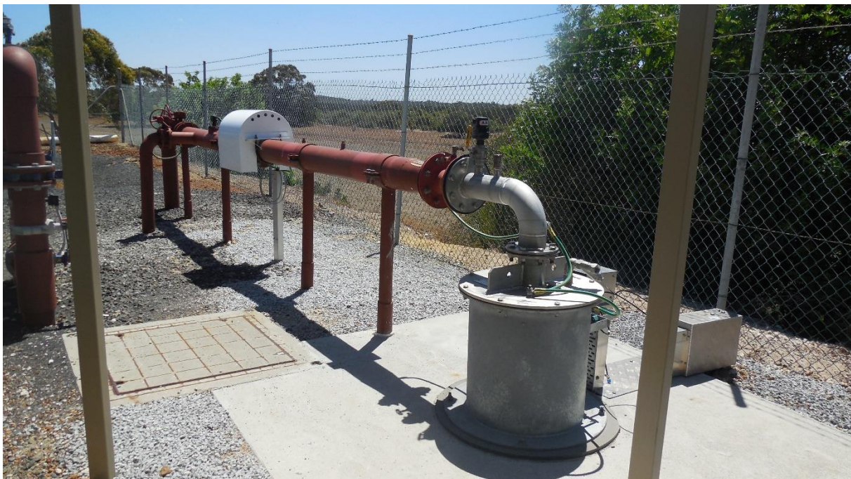
Figure C2 Confined bore 2/85 in the Town Wellfield
