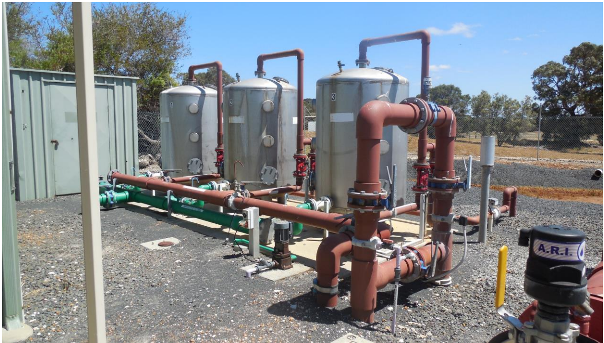
Figure C4 Media filtration is the second level of treatment for raw water, after chlorination
