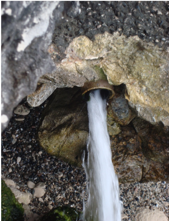
Figure C11 Pipe for discharging brine (hypersaline water) from desalination plant at Fays Bay, photograph by C. Loos
