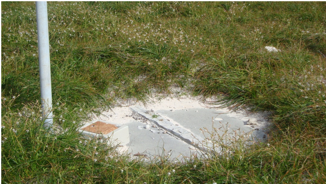
Figure C8 On-site wastewater system (septic tanks and leach drains) in Wadjemup bore field, photograph by C. Loos
