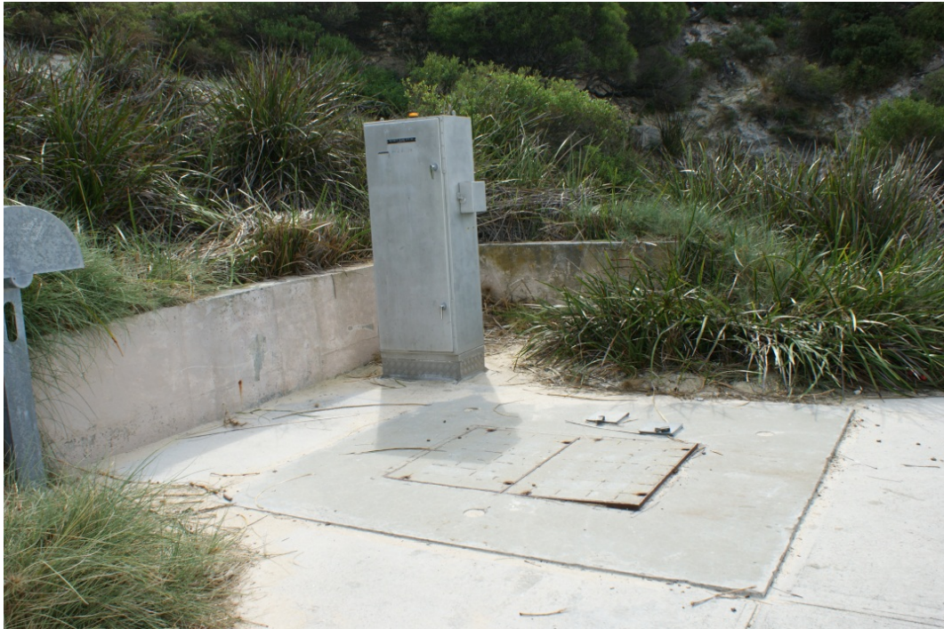
Figure C5 Sewer pump station at Longreach Bay, photograph by C. Loos
