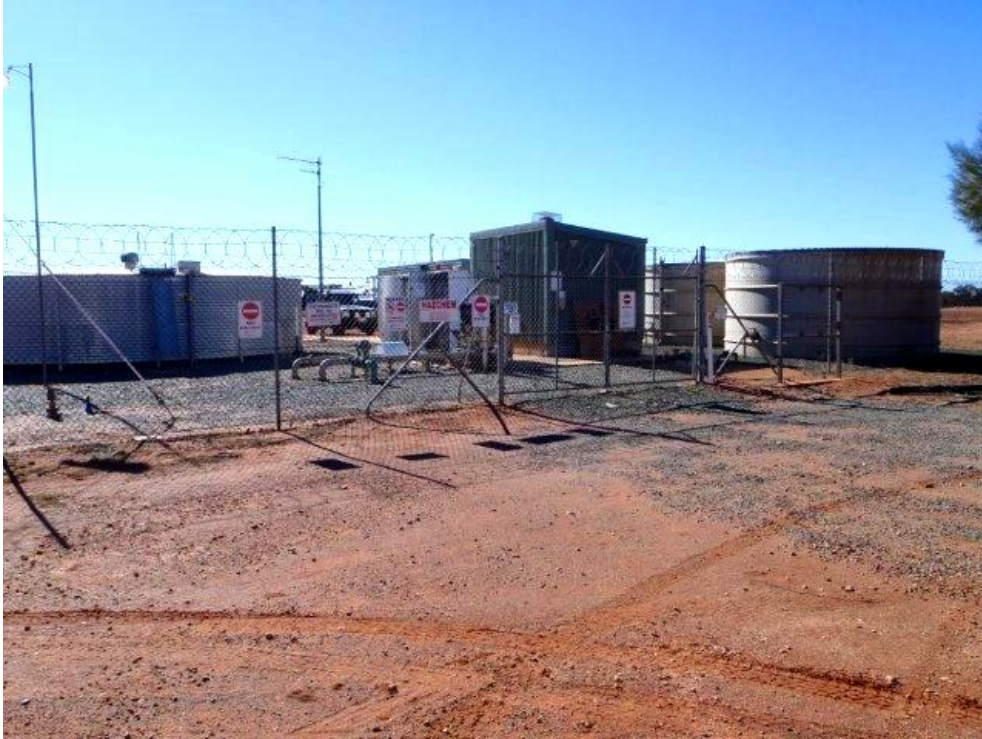
Figure C3 Wiluna Water Reserve drinking water treatment plant, photograph by M. Sawyer, Water Corporation, reproduced with permission
