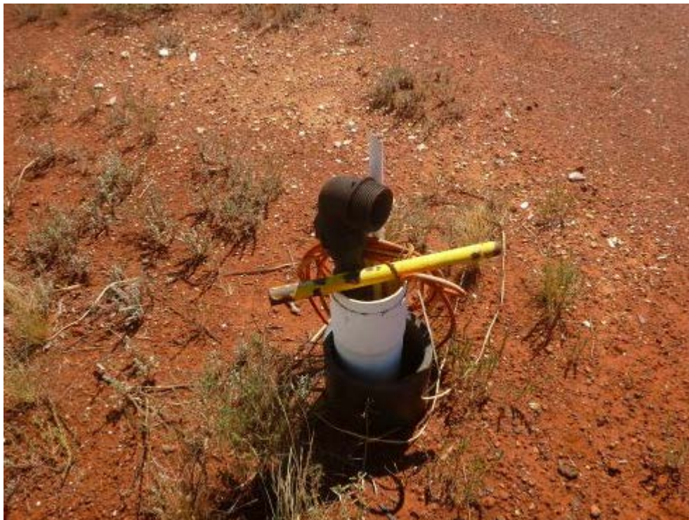
Figure C6 Unsealed abandoned bore within the Wiluna Water Reserve, photograph by H. Merrett, Water Corporation, reproduced with permission
