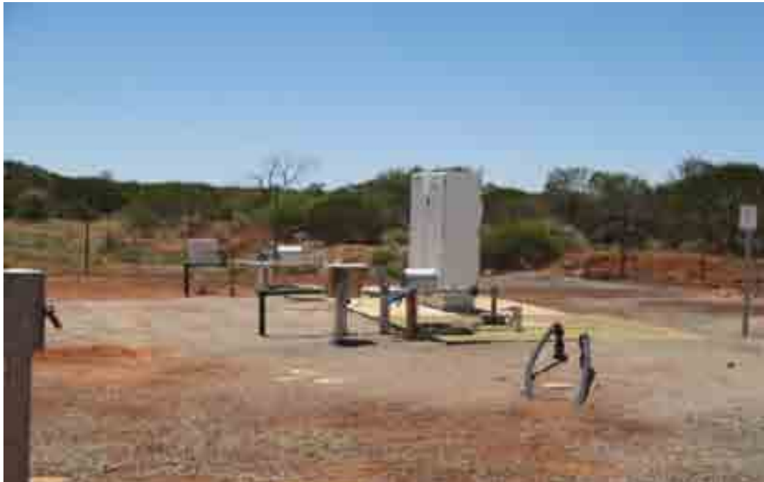
Photo 7 Bore 1/84 and 2/83 are located within the same compound as the treatment plant.
