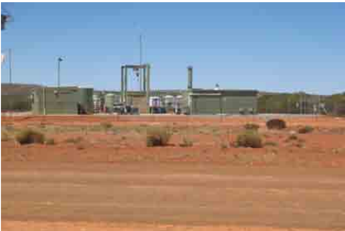
Photo 6 The unsealed Yalgoo North Road (foreground) runs close to the Yalgoo drinking water treatment plant (background).
