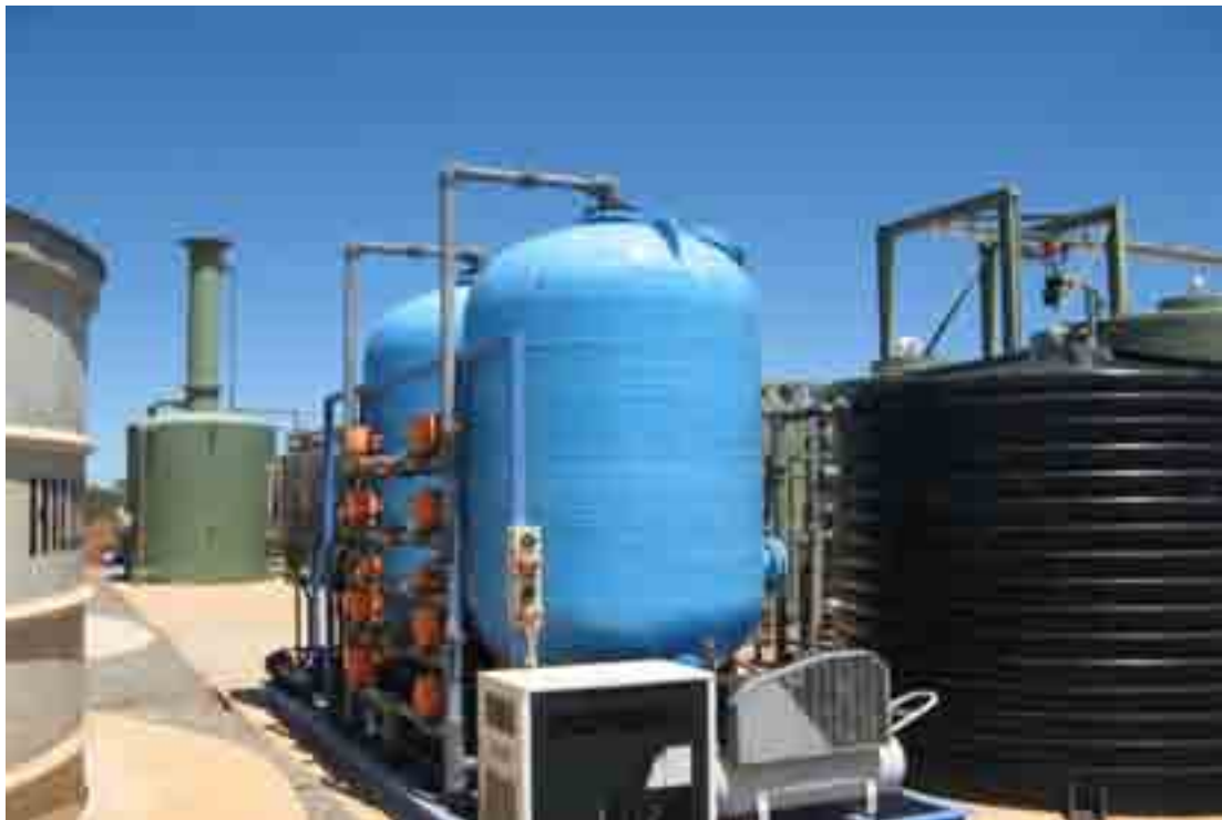
Photo 8 Inside Yalgoo drinking water treatment plant facility.
