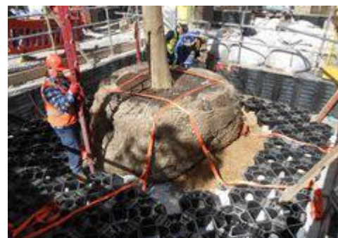
A Tree being planted with root cells around it, the pavement is then installed around the tree, over the cells
