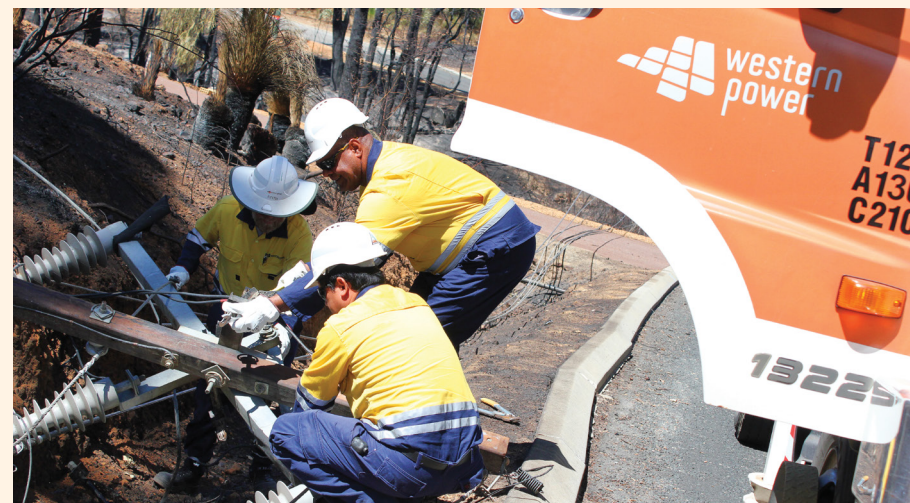
Figure 4.6 – Western Power crews assessing damage to their infrastructure following the Parkerville Stoneville Mt Helena Bushfires in January 2014
