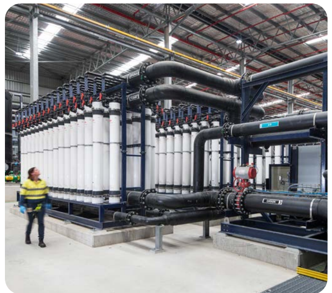
Groundwater replenishment scheme Stage 2 expansion – Water Corporation advanced water recycling plant.
