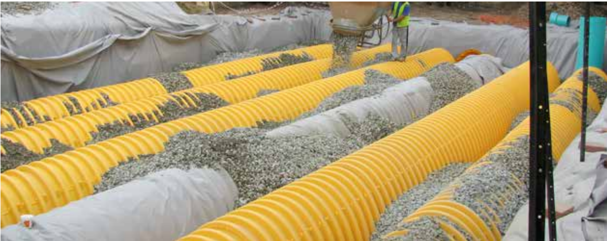
Figure 8 An example of an alternative water source – the stormwater harvesting system being built at the Graham Heal Reserve (courtesy of the City of Mandurah)
