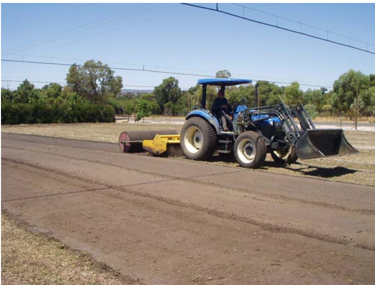
Figure 8. Palmetto soft leaf buffalo grass runners were planted into the surface 5 cm of the soil using a rotary hoe fitted with a roller.
