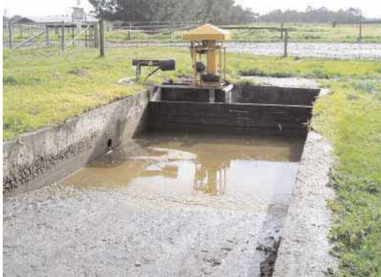
Photo 16: Trafficable sump with Rankin pump at the Vasse Research Station (courtesy Rob Summers, Department of Agriculture and Food).
