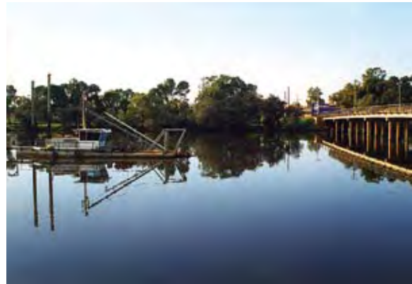
Dredge in Northam Town Pool downstream of the Peel Street Bridge, August 2000 (Photo courtesy Martin Revell)
