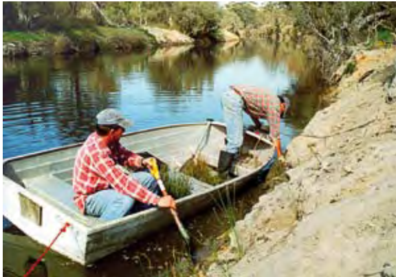
Revegetation work on the edge of Boyagarra Pool to stabilise the banks (Photo courtesy Brendan Oversby)
