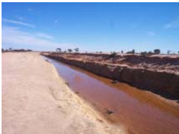
Figure 6: A main drain silted up due to spoil bank slumping and erosion
