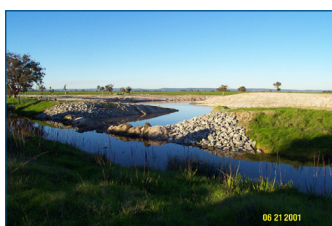
Artificial wetland entrance – 2001 Punrak Drain, upstream of 614094
