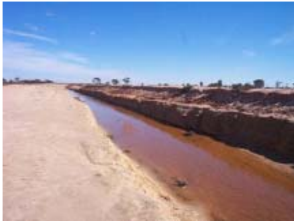
Figure 6: A main drain silted up due to spoil bank slumping and erosion
