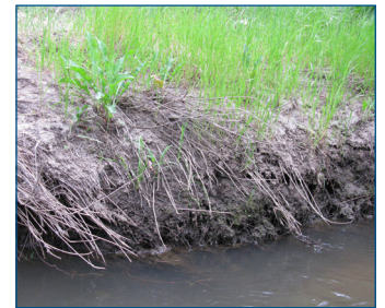
Erosion along Waroona Drain – October 2009
