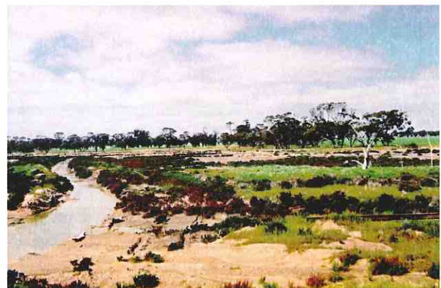
The same site in 2002, post works showing the constructed drainage and the return of vegetation (photo Catherine MacCallum)
