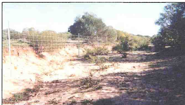
Photograph 14: Fence too close to the floodway which was not protected from washouts in large flows
