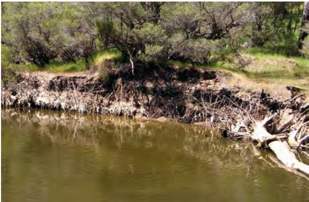
Photo 6 Bank erosion in section LA01
