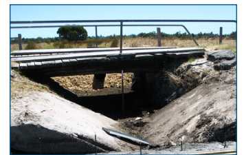
Before construction of the weir on Gull Road Drain (downstream view February 2005)
