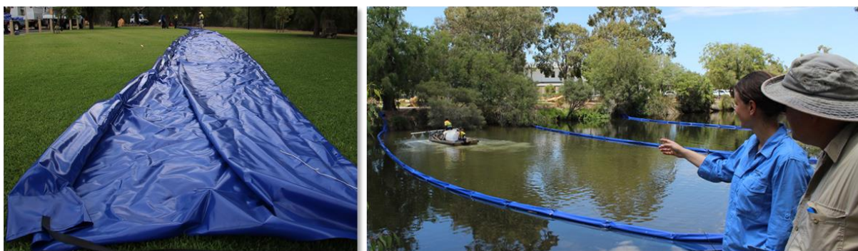
Figure 5: Floating curtains installed in the Lower Vasse River for the 2017–18 HT-clay trial.
