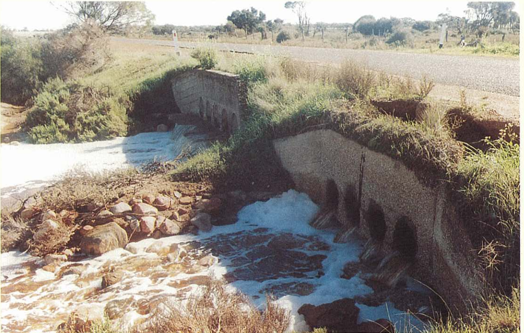
ROAD CULVERTS SOMEWHERE IN THE MOORE RIVER CATCHMENT. NOTE HOW THE PIPES ARE RAISED ABOVE THE BED LEVEL. IT IS IMPOSSIBLE FOR SMALL FISH TO MOVE UPSTREAM THROUGH THESE CULVERTS. PHOTO: P. MUIRDEN
