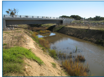
In-stream vegetation downstream - June 2010
