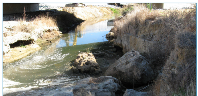
Erosion and bank undercutting – May 2009
