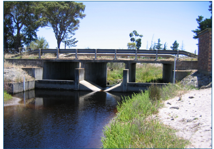
Meredith Drain, Johnston Road – December 2006
