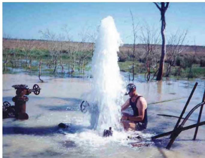
Water supply out of control
