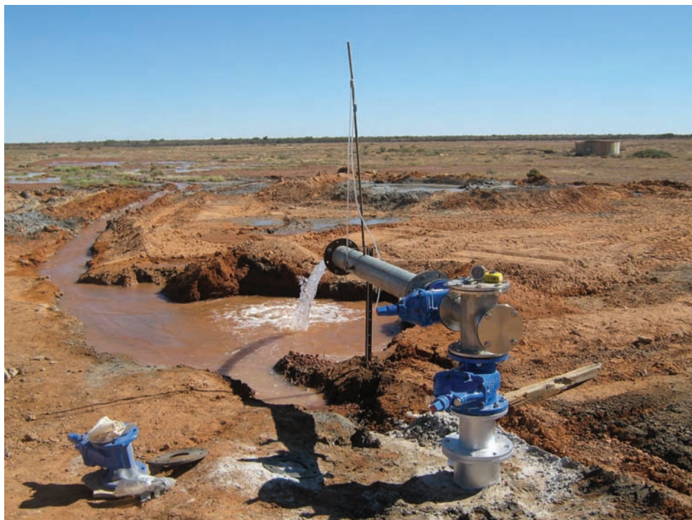
Flowing artesian bore (prior to site cleanup)
