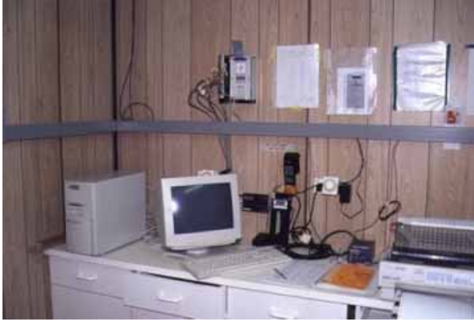
Figure 3.13 Karratha MS - data logger and communications equipment.
