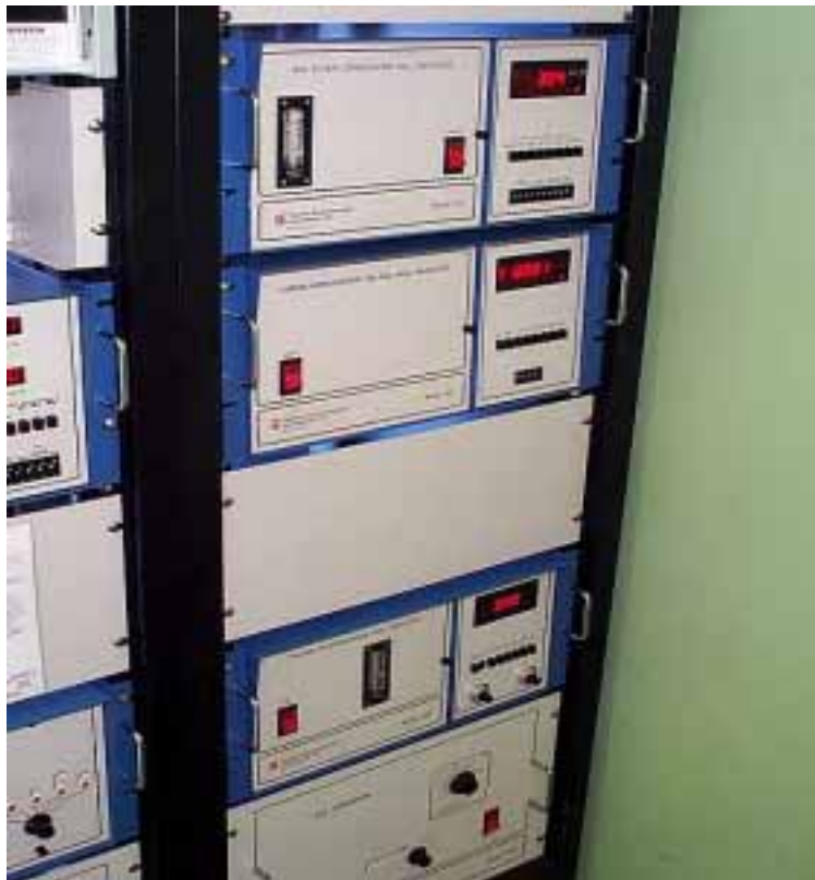
Figure 3.6 King Bay AQMS - gas analysers.
