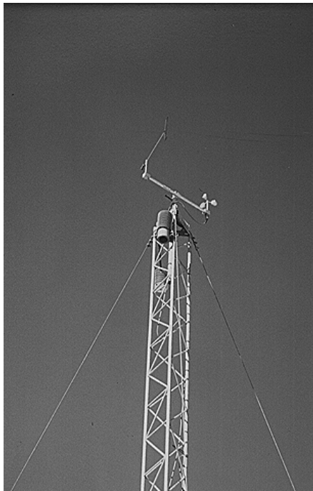
Figure 6.1 - Meteorological equipment on a 10 metre guyed tower.
