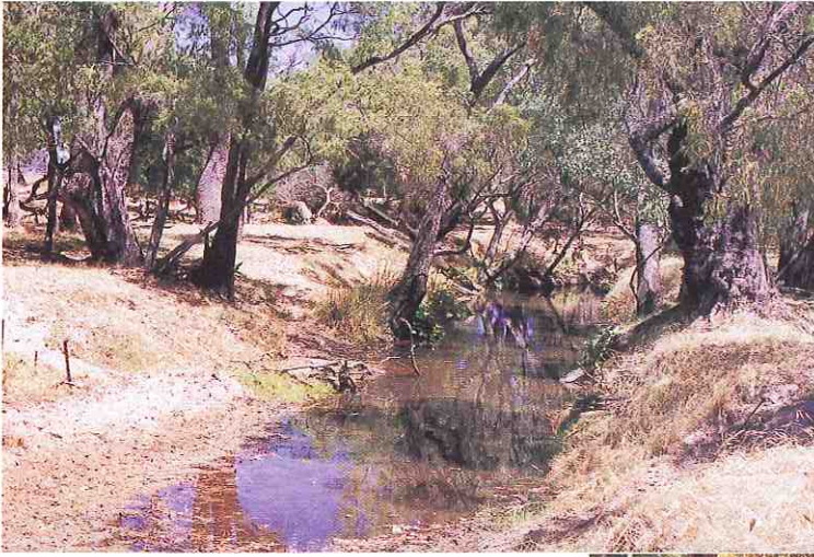
C1-C2 grade foreshore on the Sabina River. Trees remain though there is little evidence of regeneration. The shallow-rooted weedy understorey provides no support to the soil, making the banks vulnerable to erosion.
