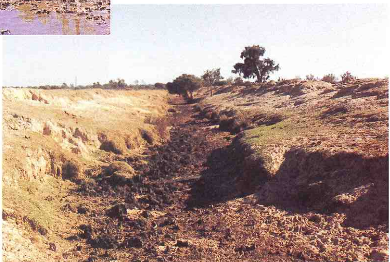
D2 grade foreshore on the Abba River. No vegetation remains to control erosion. The sandy banks are actively eroding and contributing to the accumulation of sediment downstream.
