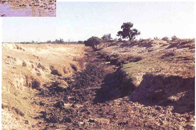
D2 grade foreshore on the Abba River. No vegetation remains to control erosion. The sandy banks are actively eroding and contributing to the accumulation of sediment downstream.
