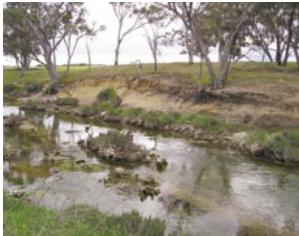
Photo 3: Erosion of 'sand lens' intersected by the river in Photo Section 11
